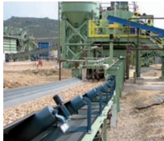
Overland conveyor feed end at the Kisladag property
